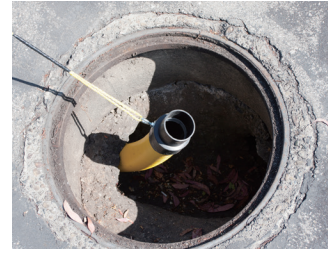
Tiger tail used on a manhole
